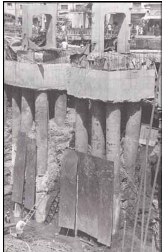
Figure 14. Vertical bored piles installed in hard rock as raker pile ( rake 1 H in 5 V )
