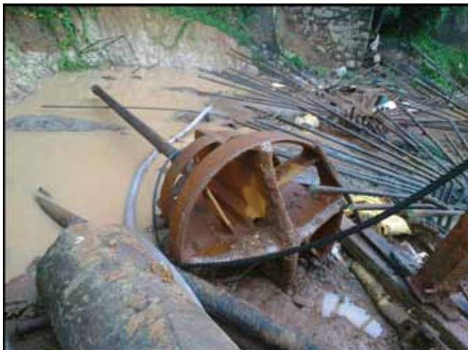
Figure 12. Rock cutting chisel of sub-standard quality in use.
