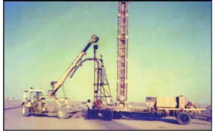
Figure 5. Set-up for pumping concrete from Transit Mixer to pile tube at a height.
