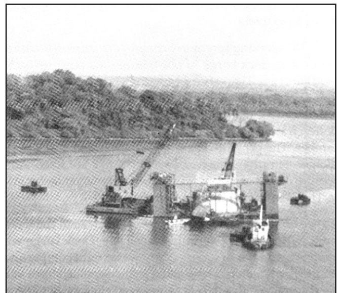
Figure 4. A view showing sinking of caisson in progress for the Zuari bridge
