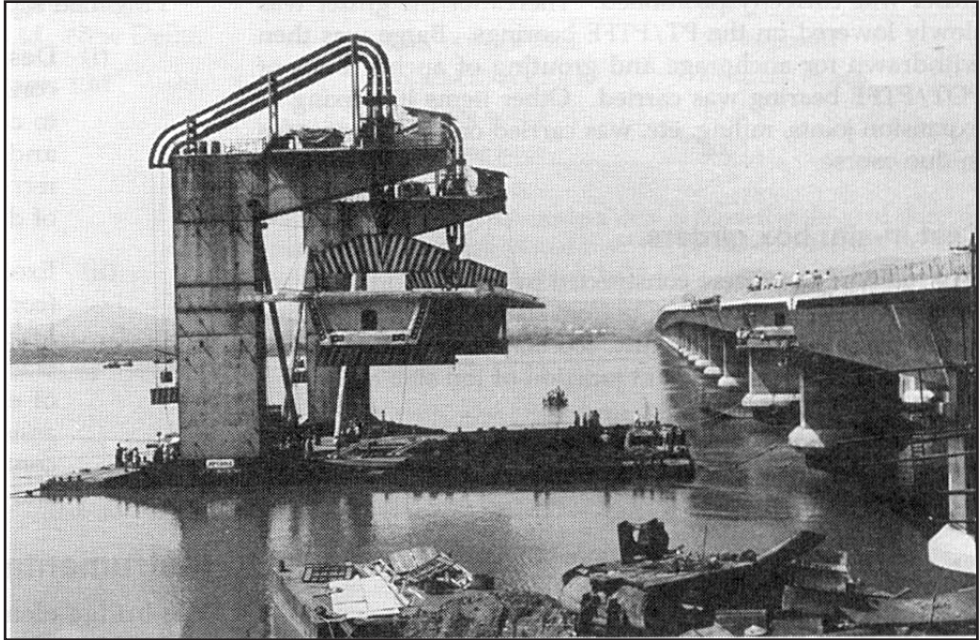
Figure 4. Girder being lifted up by hydraulic jacks and towed to bridge location
