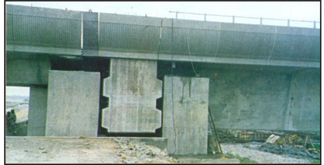
View showing extended portion of end diaphragm of box girder sandwiched between concrete stoppers
