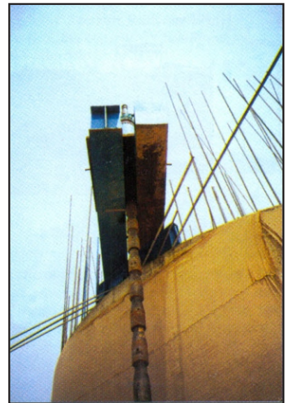
Gripper rod passing through cross beam and connected to central hole jack at top
