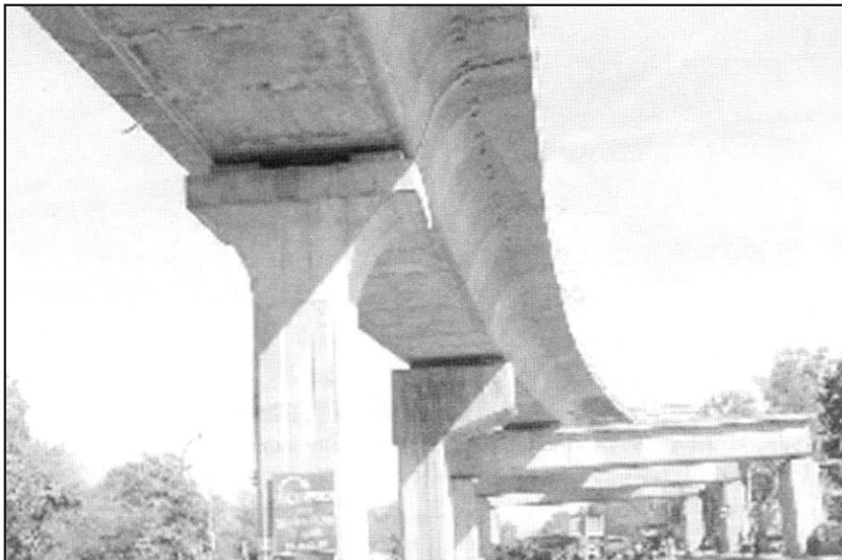
Figure 10. Precast segmental viaduct for Delhi Metro; note that the portals and different pier shapes were required as alignment traverses from side of road to its centre
