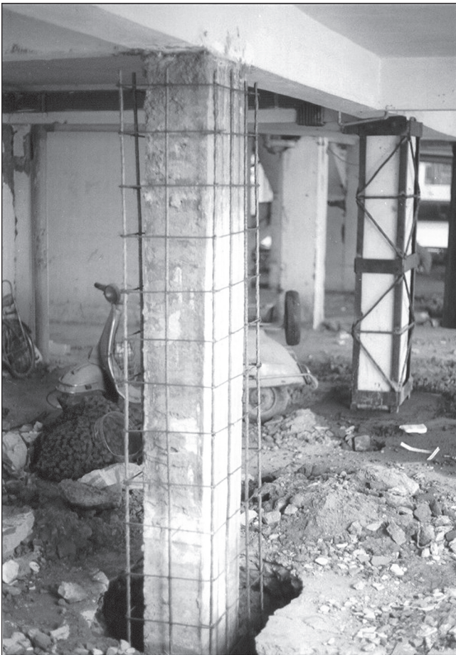
Figure A. Inadequate strengthening of columns
