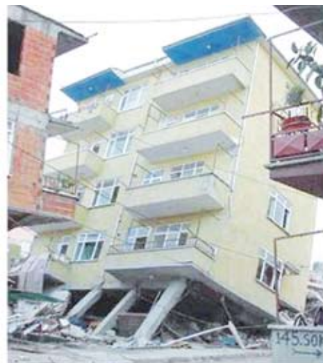
(b) Soft storey failure in M 7.4 earthquake, Turkey, Aug. 17, 1999
