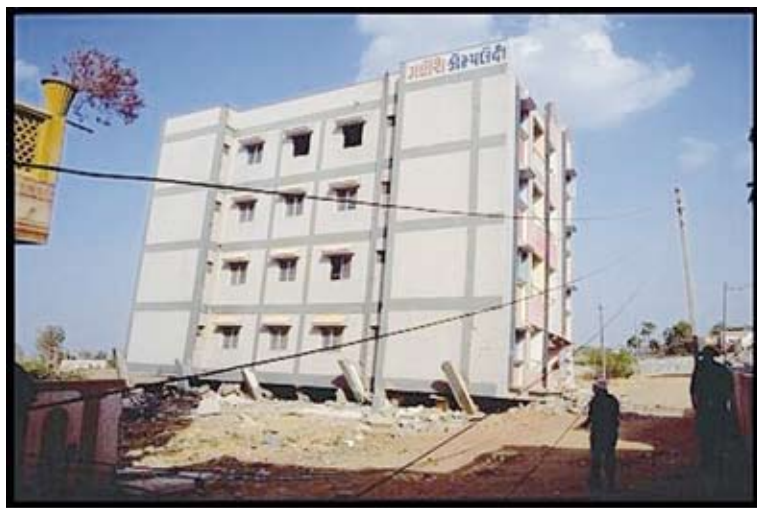
(a) Soft storey failure during the M 7.7 earthquake, Gujarat India, Jan. 26, 2001
