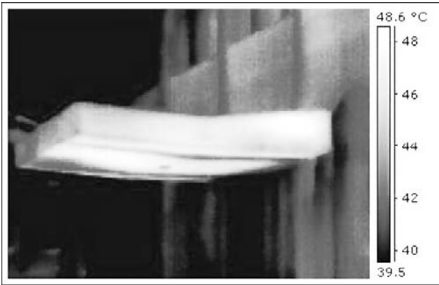
Figure 3. Moisture penetration in a canopy
