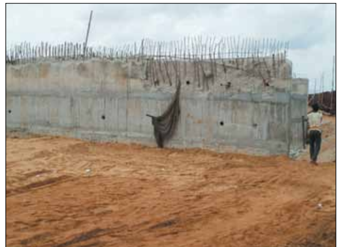
Figure 4. Damaged wall pier after collapse of staging for a subway roof slab
