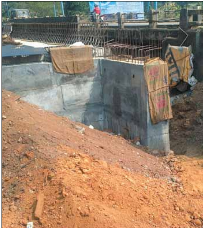
Figure 10. Poor quality curing for abutment and return wall
