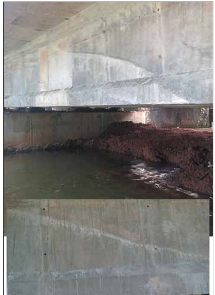
Figure 5. Cold joint formation in a deep bridge girder
