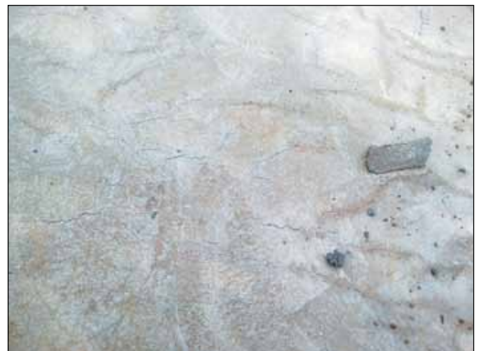
Figure 8. Multiple cracks on top of a deck slab
