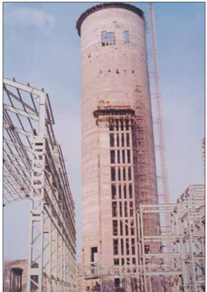
Figure 2. Urea prilling tower built using slipform at a fertiliser plant in U.P
