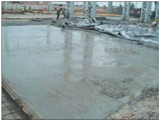
Figure 6. Finished concrete surface with bleeding water unattended
