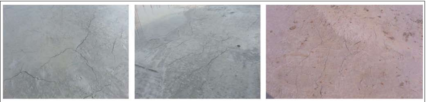
Figure 1. Cracks after concrete casting
