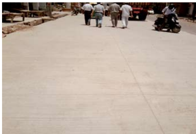
Figure 1. A typical surface of the constructed portion of a conventional white-topping over existing distressed bituminous road in Delhi
