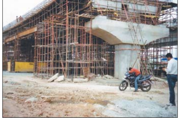
Figure 5. Sample of staging meant to carry heavy load from cast-in-situ deck superstructure
