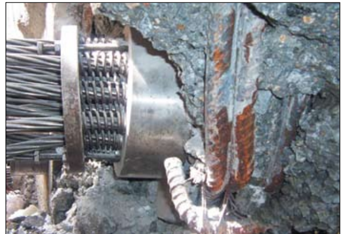
Figure 3. Unsound concrete in end block of a PSC girder
