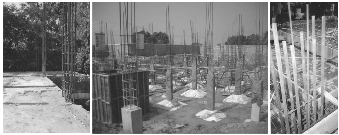
Figure 1. Columns not properly designed or executed: (a) Kinking of longitudinal bars, (b) Insufficient curing, (c) Minimal transverse reinforcement
