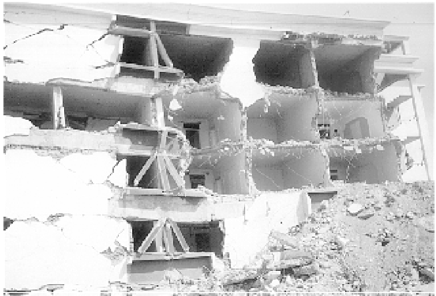
An inadequately designed hotel building collapsed during the Bhuj earthquake. The hotel was inaugurated in December 2000 and collapsed on January 26, 2001
