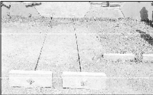
Fig 3 Anchored earth system with metallic bars and anchor blocks, licenees: MBN Anchored Earth Ltd
