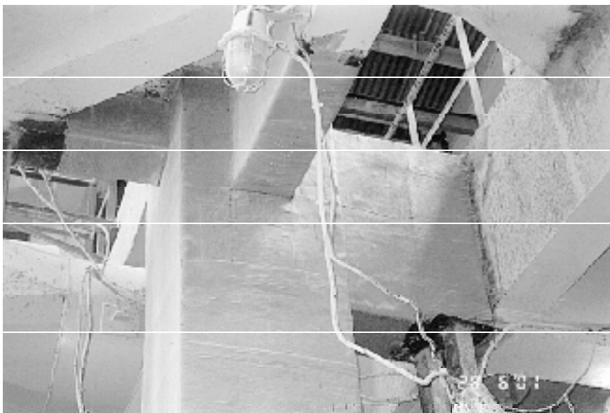
Retrofitted joint of an earthquake-damaged industrial structure, Gujarat
