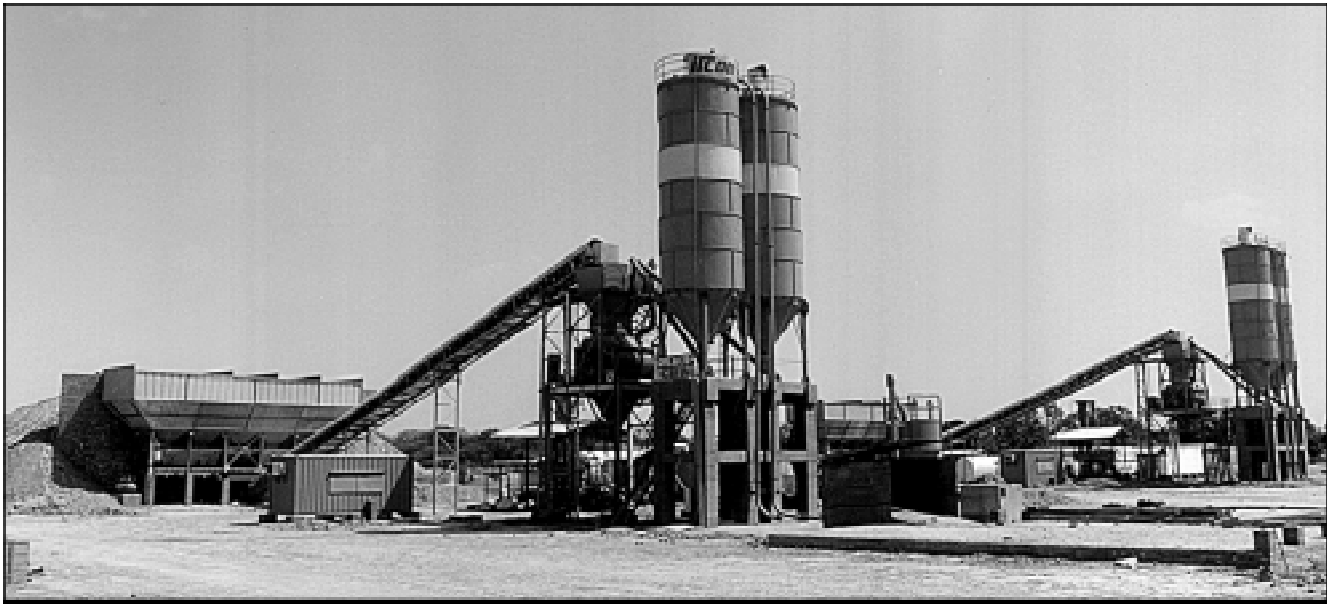
"Personal 45" CIFA-Greaves batching plant at project, NH-2 package III C road project, Allahabad
